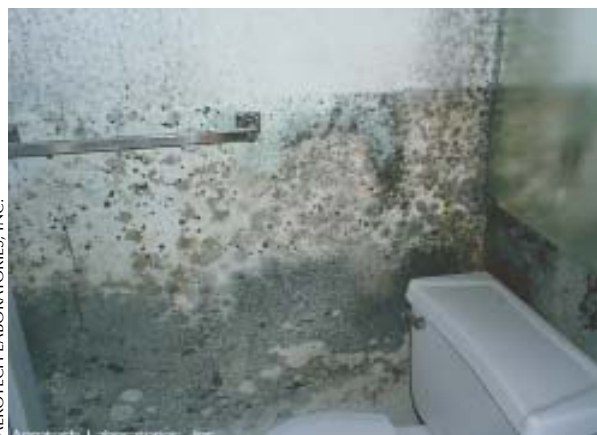
Figure 5. The bathroom is a naturally humid environment and is also prone to plumbing leaks that create continual wet conditions. Drywall, whether moisture resistant or not, supports thriving mold colonies in moist conditions. Use backerboard and tile instead, or a synthetic material like solid surfacing.
