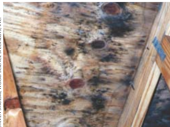
Figure 6. A dryer vent and bath fan were improperly vented into this attic, causing condensation to form on the sheathing and support mold growth.
