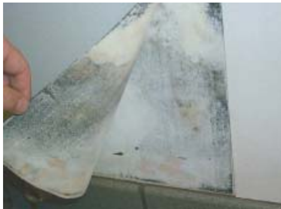
Figure 4. In hot, humid climates, vinyl wallpaper forms a vapor barrier on the cool, air-conditioned side of the wall, causing exterior moisture to accumulate under the wallpaper and support the growth of mold. Walls should be vapor-permeable on the side facing dry air, and vapor barriers should be placed on the side facing moist, warm air.
